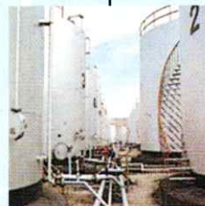
Slack-wax, Storage Tank
